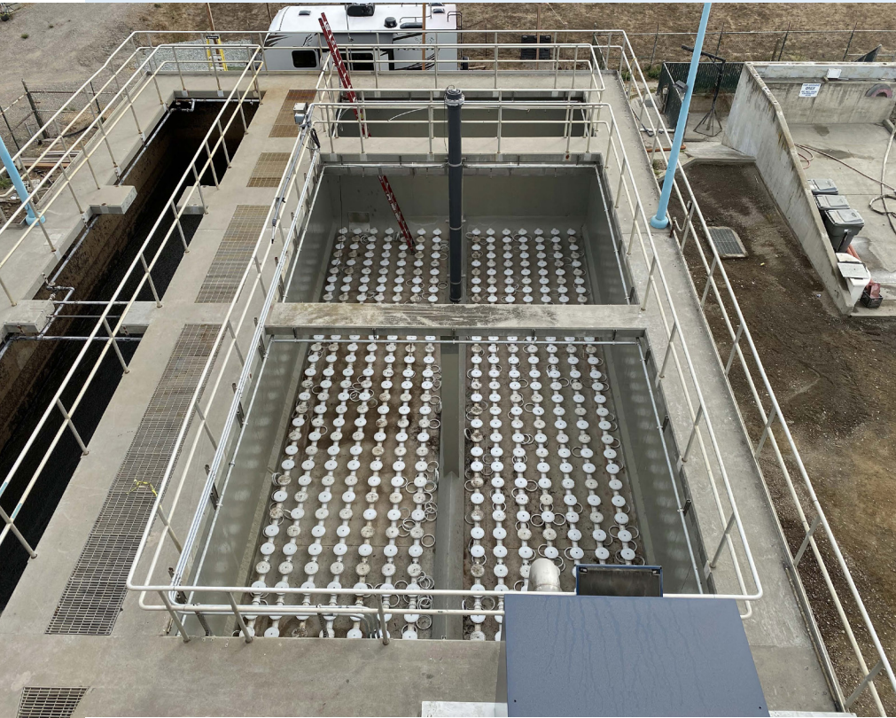
Oro Loma Sanitary District installed of a full-scale Microvi wastewater side-stream treatment system to treat nutrients at their treatment plant in San Lorenzo, CA. The innovative watershed nutrient permit for SF bay facilitated the evaluation and select
